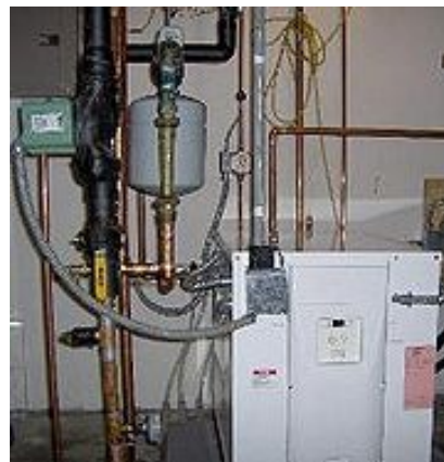
Fig.6 Water-to-water heat pump
