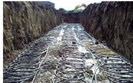
Fig.2 A 3-ton slinky loop prior to being covered with soil. The three slinky loops are running out horizontally with three straight lines returning the end of the slinky coil to the heat pump
