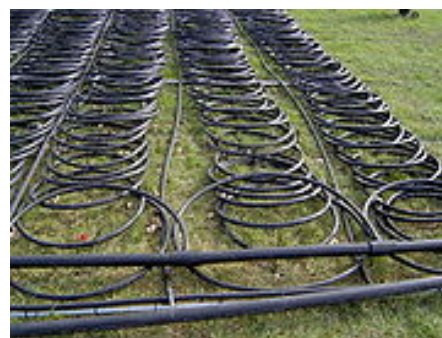
Fig.4 12-ton pond loop system being sunk to the bottom of a pond
