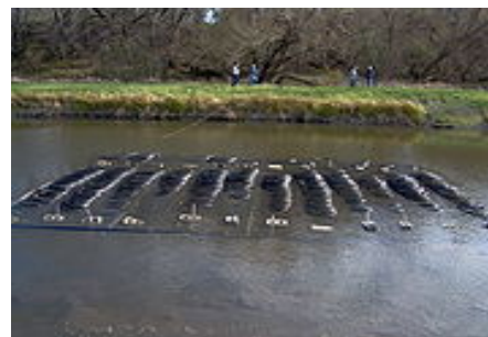
Fig.3 Loop field for a 12-ton system (unusually large for most residential applications)
