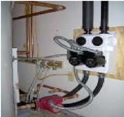
Fig.1 An installed liquid pump pack
