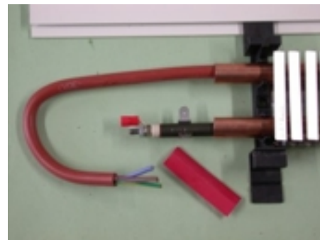
Fig. 7 Electrical plinth mounting in a house
